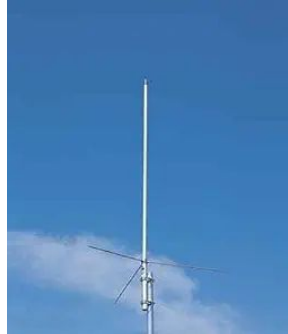
Base antenna on top of a roof
